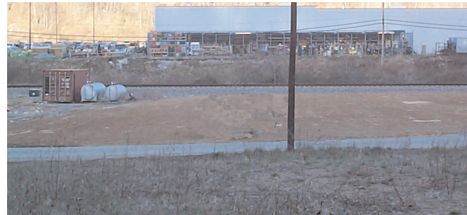
The townhouse component of Olympic Homes is currently being built on the cleared land pictured above. Harlan's Wal-Mart will be a short walk away.
